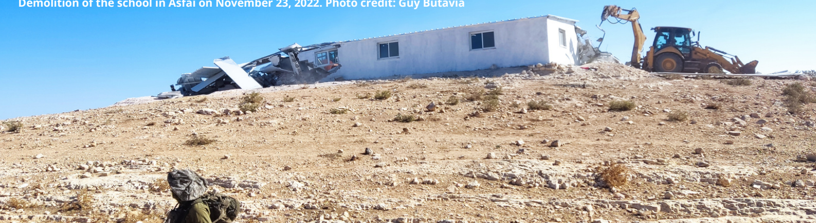
Demolition of the school in Asfai on November 23, 2022. Photo credit: Guy Butavia
